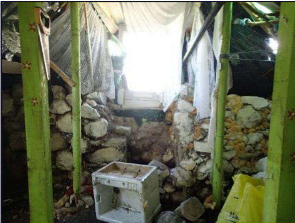
Figure 23: Hobble of fireplace built into west Gable, mostly collapsed
