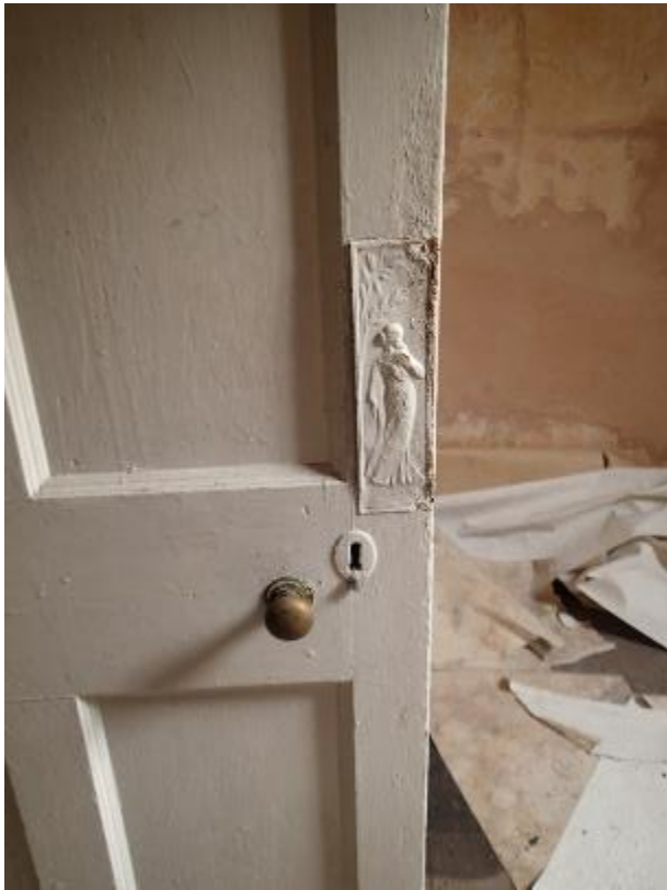
Figure 25: Decorative fingerplates on door to FF6
