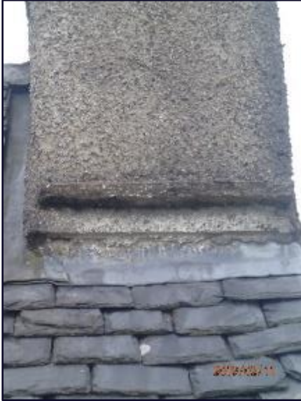
Figure 10: Weathering Slate on NW Chimney stack
