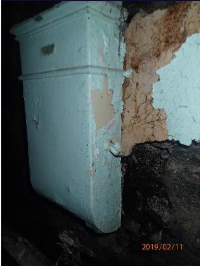
Figure 26: Wall Ventilator designed and made by Robert Boyle and sons, Glasgow
