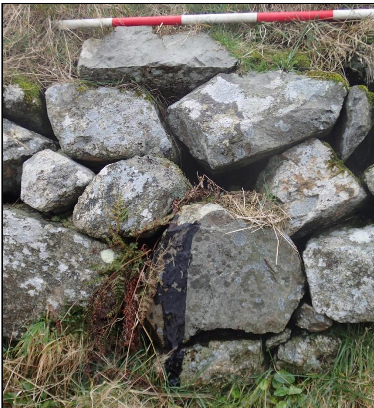
Figure 14: Tar on North Eastern external wall (003), presumably from a time after thatching when the roof was “modernised”.
