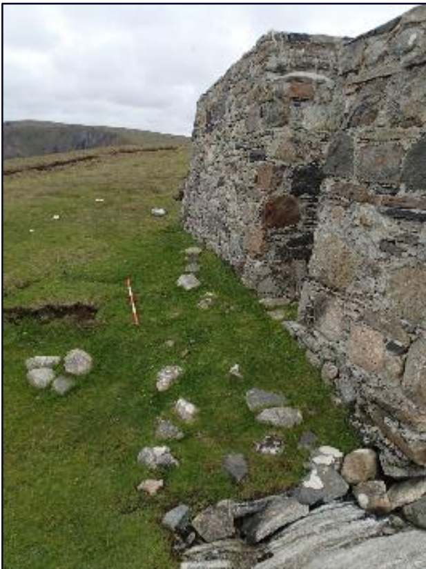
Figure 28: North side of Look out structure showing possible earlier wall at base
