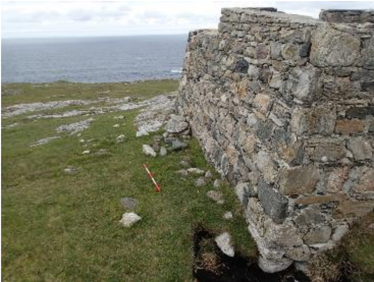
Figure 29: South side of Look out structure showing possible earlier wall at base
